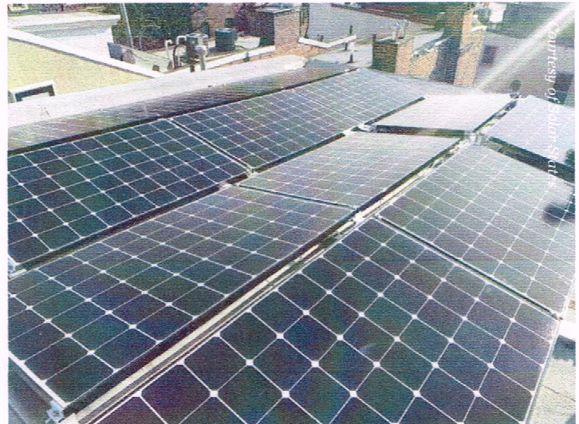
Solar panel array installed on a Center City roof.
