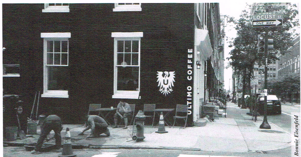
Workers repair the unpaved section of sidewalk in front of the Ultimo Coffee Bar.
